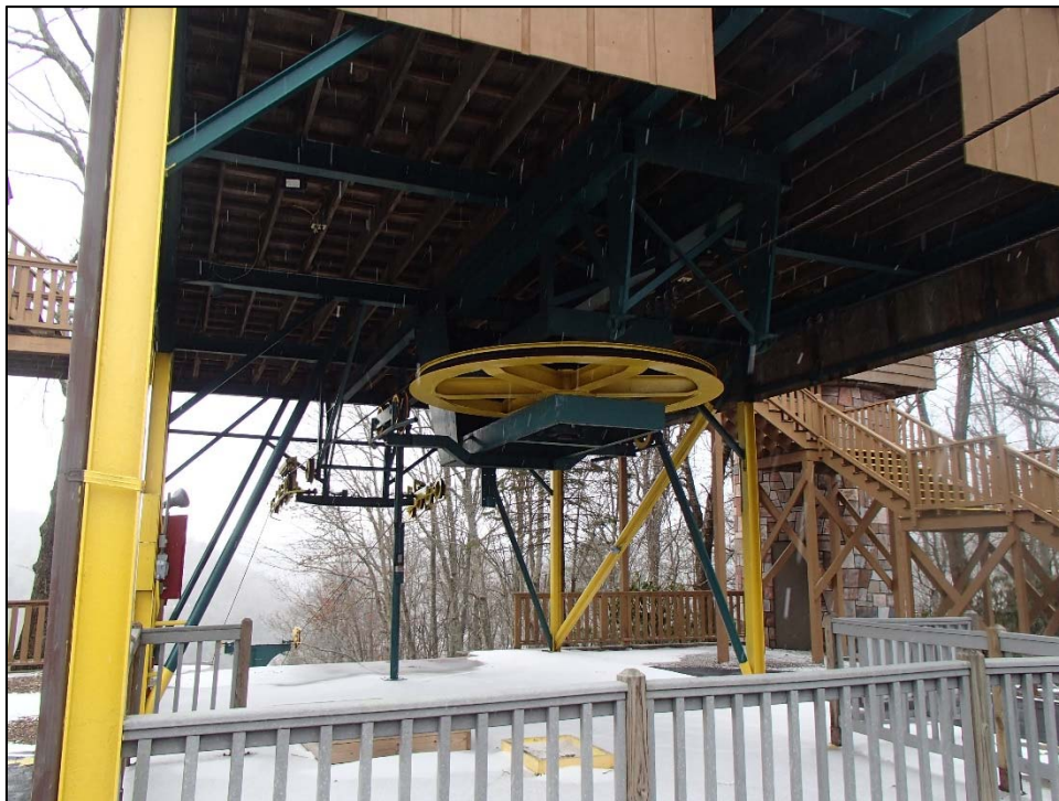
Figure 16: Chairlift Mechanical System
